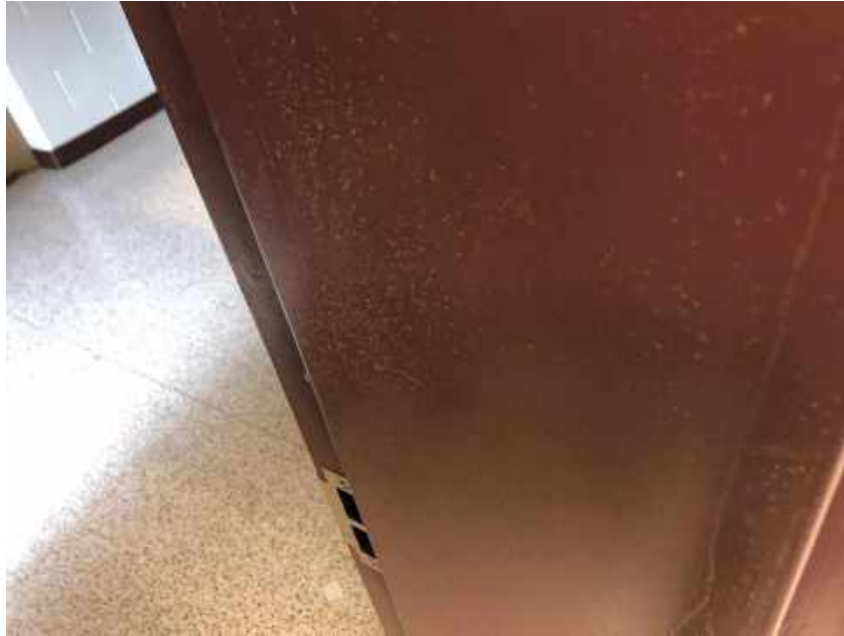
View of Microbial Growth on Metal Door Frame (Band Room 41)
