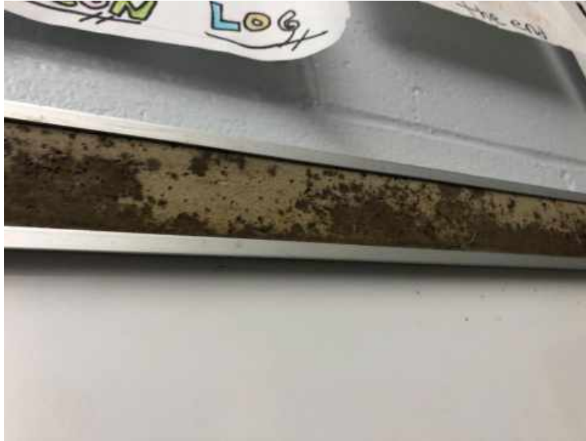
Typical View of Microbial Growth on Cork Strips Throughout Classrooms (Classroom 82)
