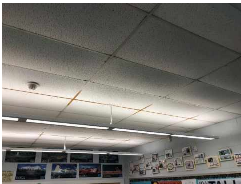
Typical View of Ceiling Tiles “Curling” and Grid Rusting Indicative of Historically Humid Conditions (Classroom 85)
