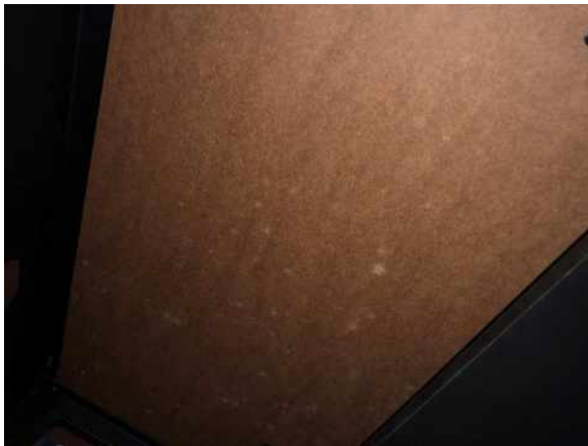
Typical View of Sporadic Minor Growth underneath Tables (Library Computer Lab)
