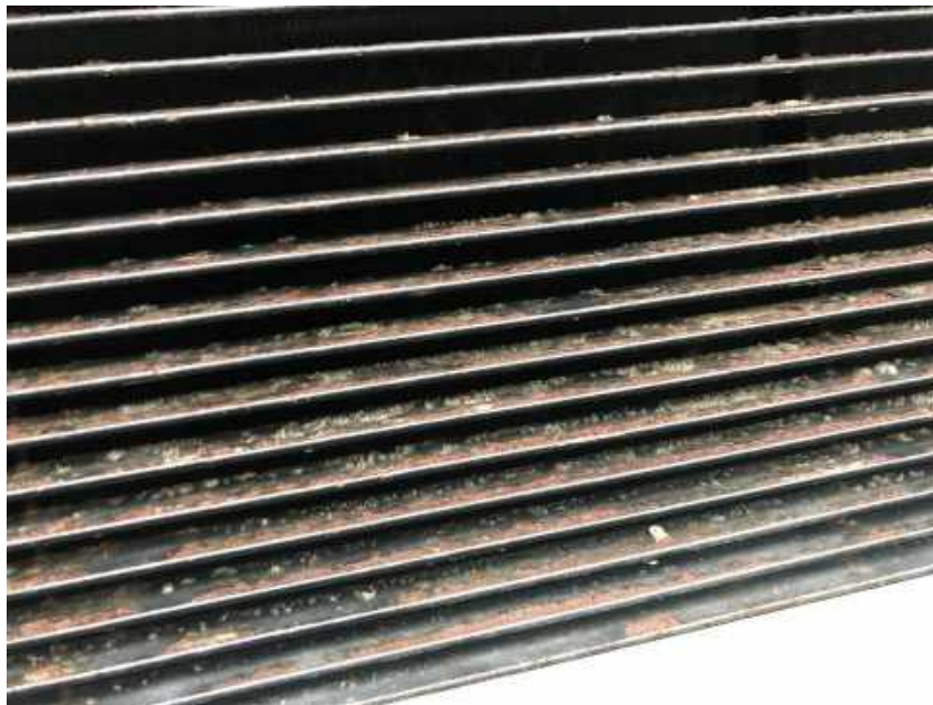
Typical View of Microbial Growth in HVAC Univent within Classrooms (Classroom 11)
